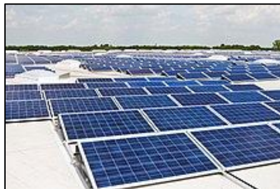
FIGURE 3: ARRAY OF SOLAR PANELS
